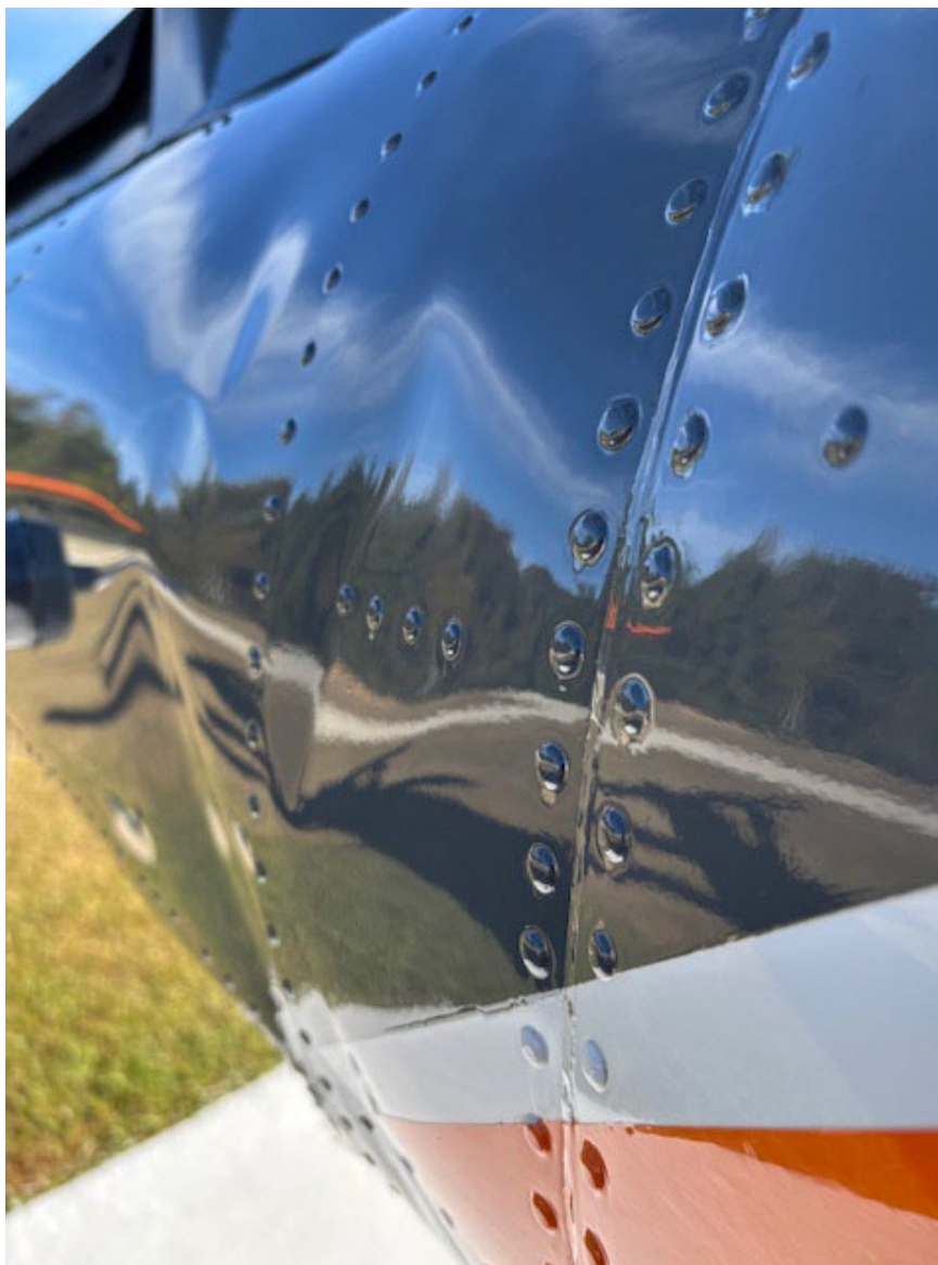
Photograph 3 - Damage to Right side of Tail boom (Courtesy of Oprerator)
