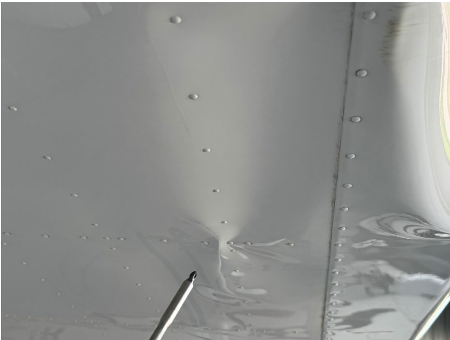
Photograph 5 - View of underside of right-hand wing showing buckling from spar damage (Courtesy of Maintenance Facility)
