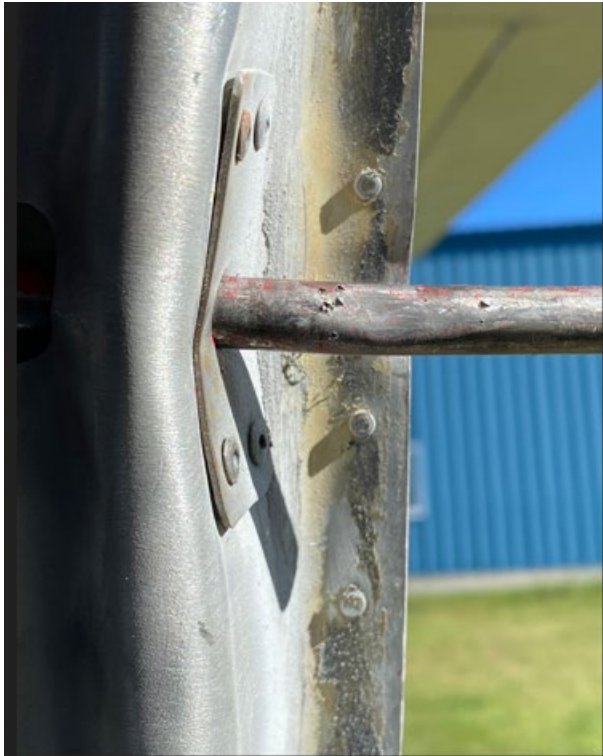
Damaged Locking Rod and Door Structure located at the Trailing Edge of Door.
