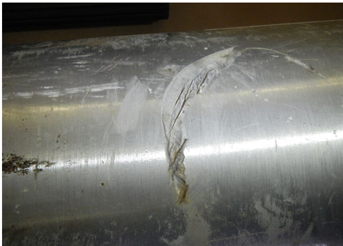
Figure 2: Cylinder #1, exterior wall gouge (March 26, 2025).
