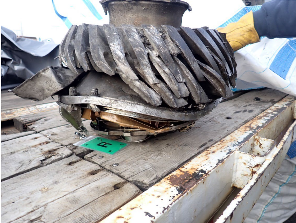
Figure 54: Fan Assembly 1 Side View of Damaged Disk (Courtesy of Honeywell)
