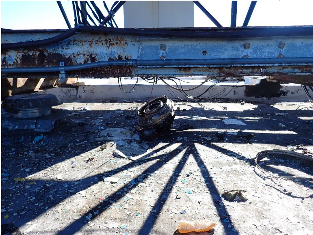
Figure 57: Fan Assembly 2 on Roof of Commercial Building (Courtesy of Honeywell)
