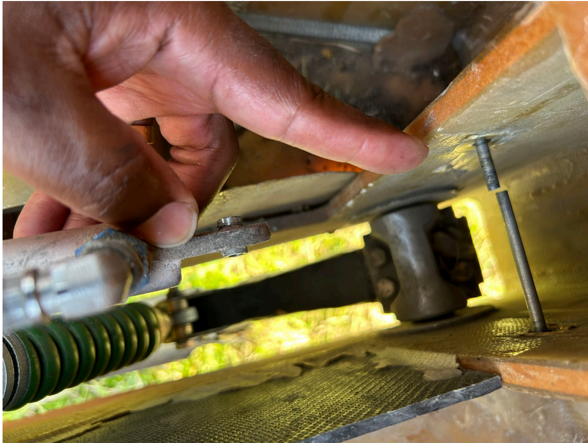
Photograph 2 - View of broken actuator bolt. (Courtesy of FAA)
