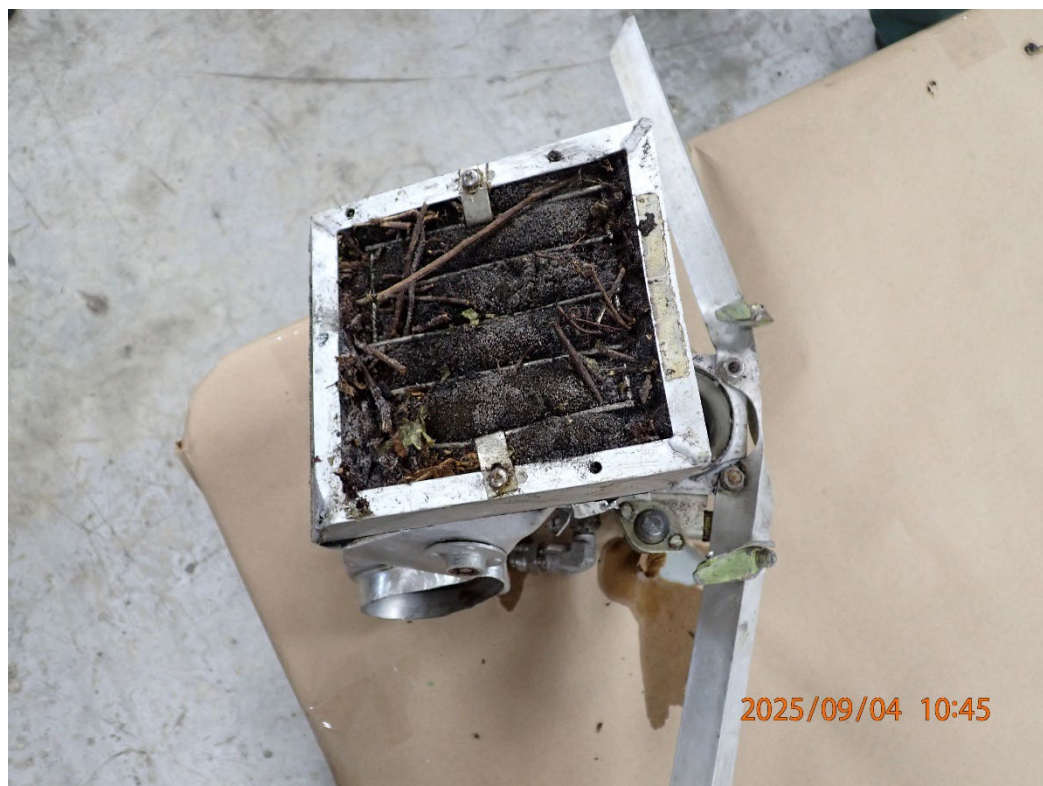
Photo 21: View of the air intake filter.
