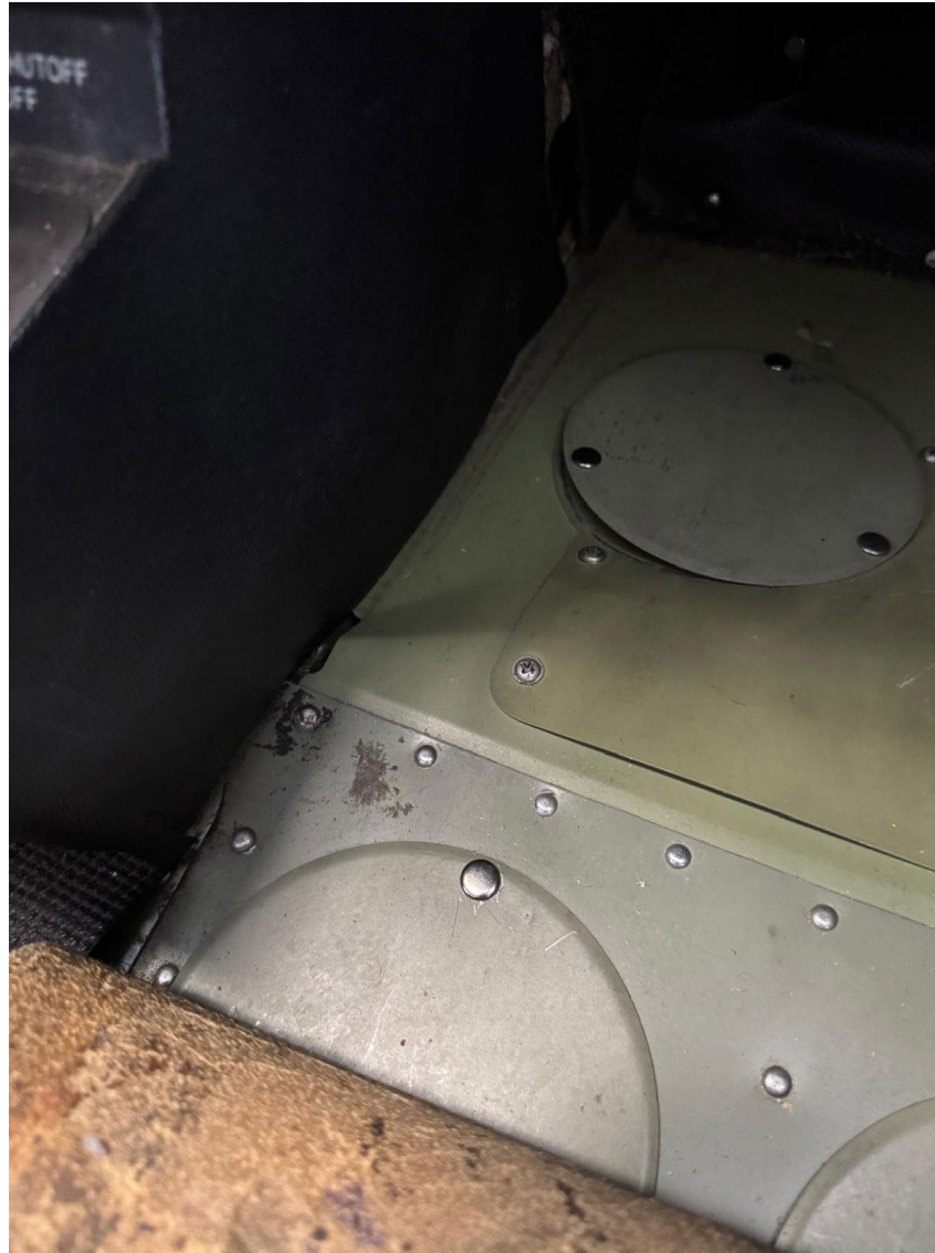
Photograph 2 - Floor Damage (Courtesy of FAA)
