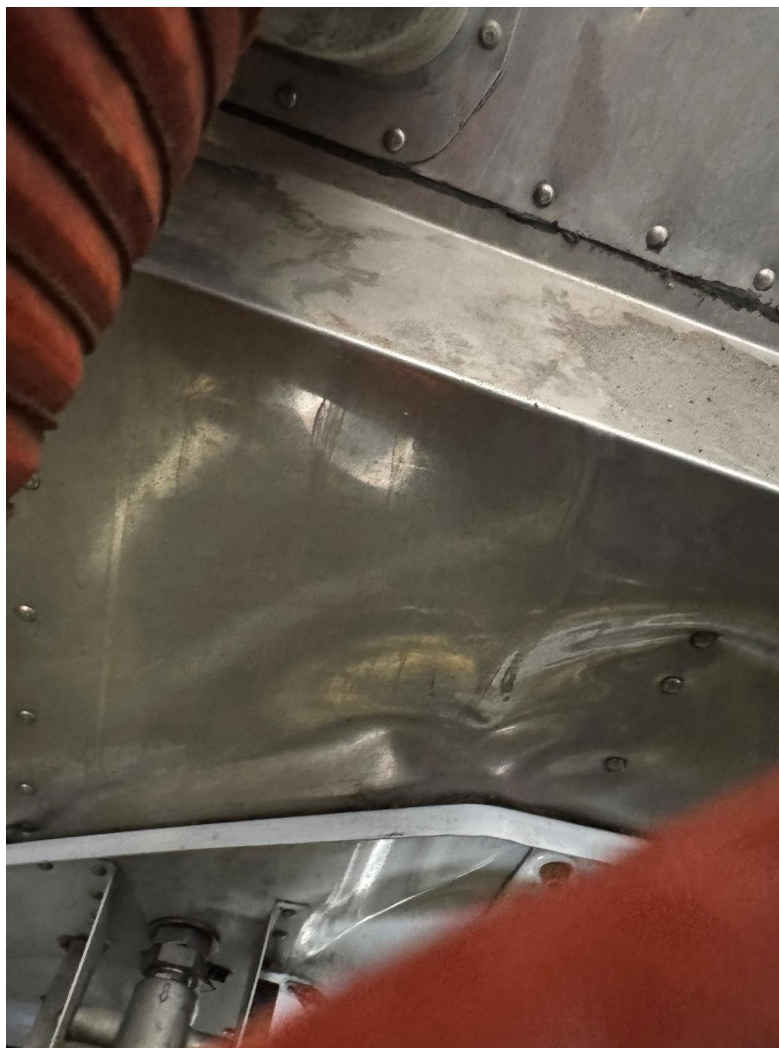
Photograph 1 - Firewall Damage (Courtesy of FAA)
