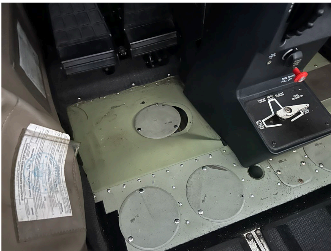
Photograph 3 - Cockpit Floor Buckling Damage (Courtesy of FAA)
