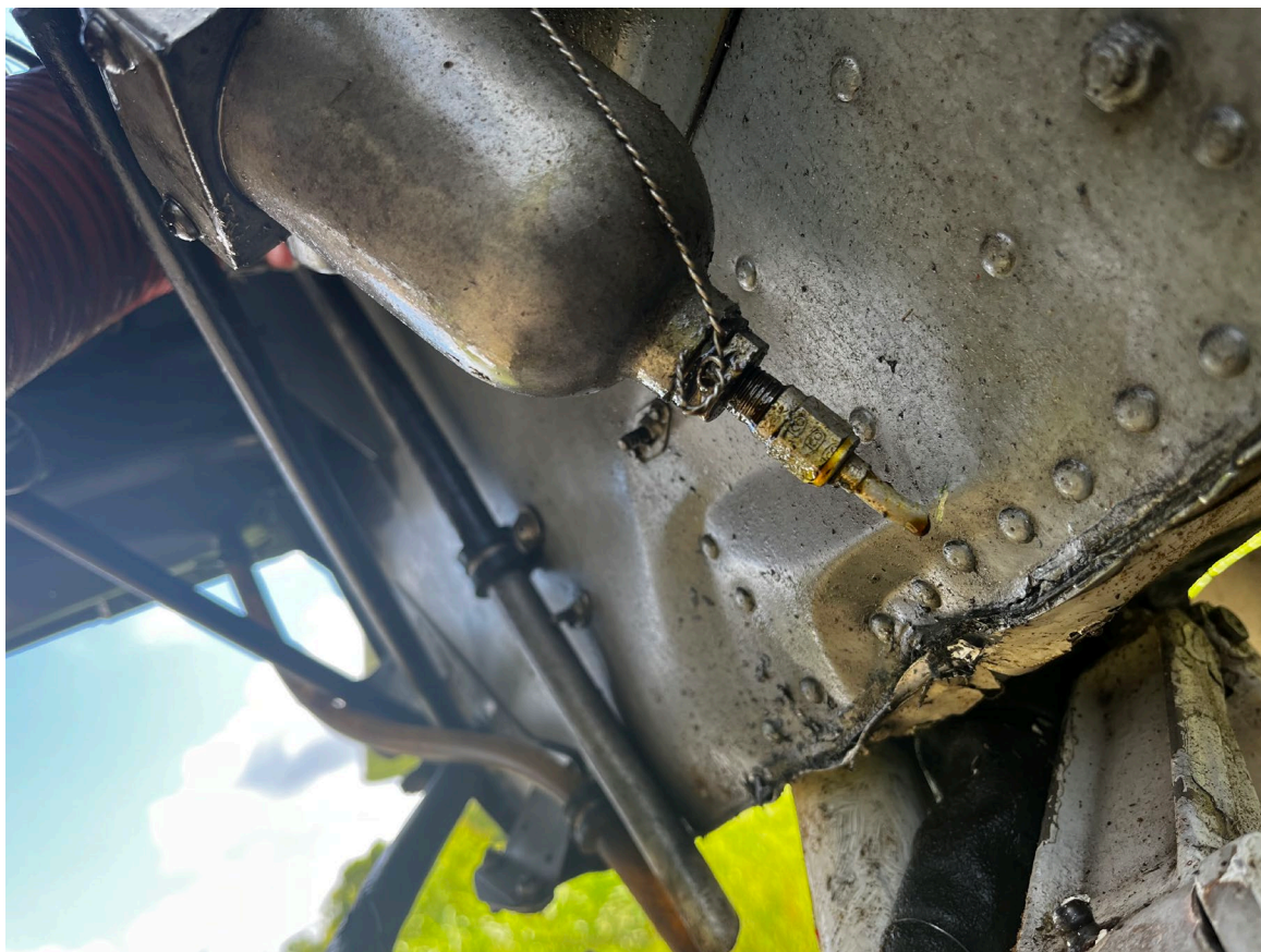
Photograph 4 - Lower Firewall (Courtesy of FAA)
