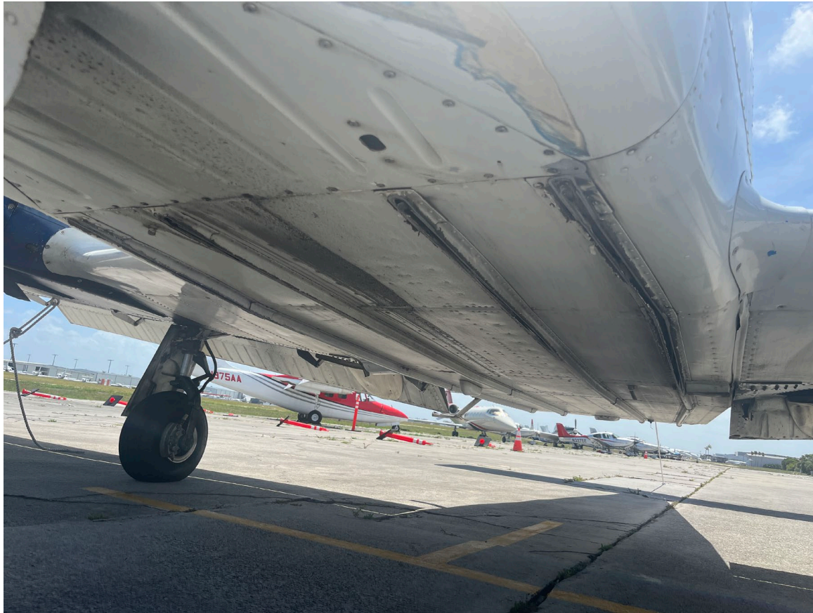
Photograph 5 - View of the Fuselage Bottom Noting Damage to External Longerons (Courtesy of FAA)
