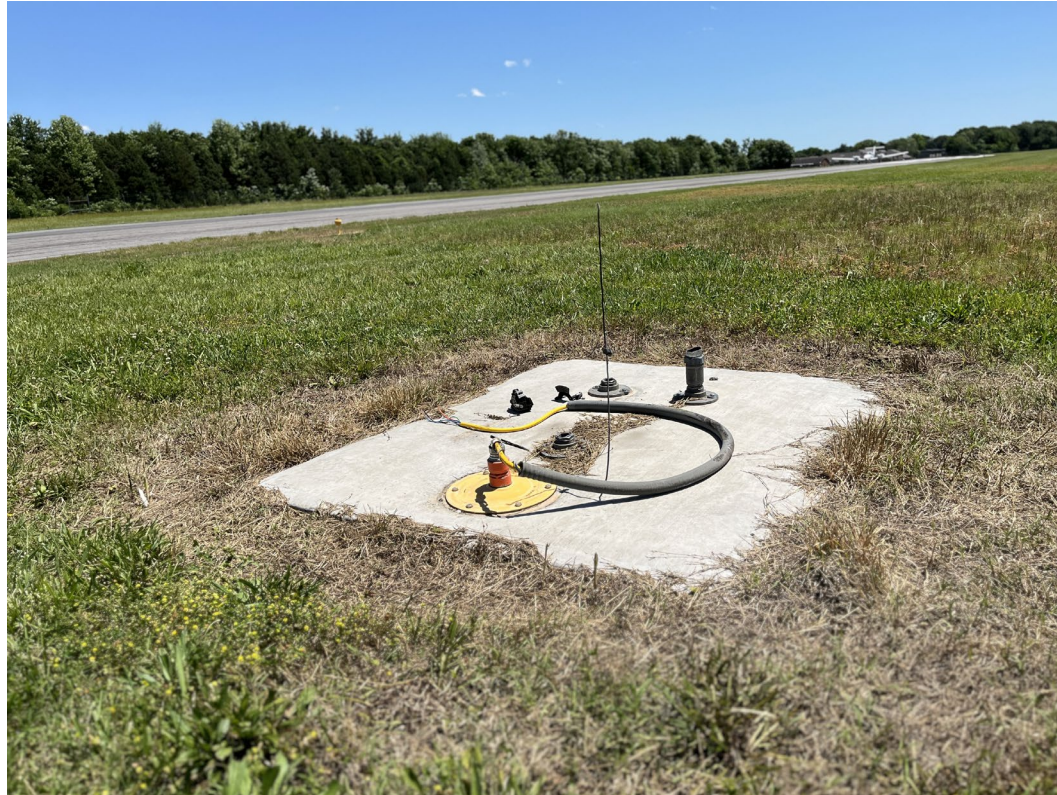
Photograph 4 - View of damaged runway light. (Courtesy of FAA)
