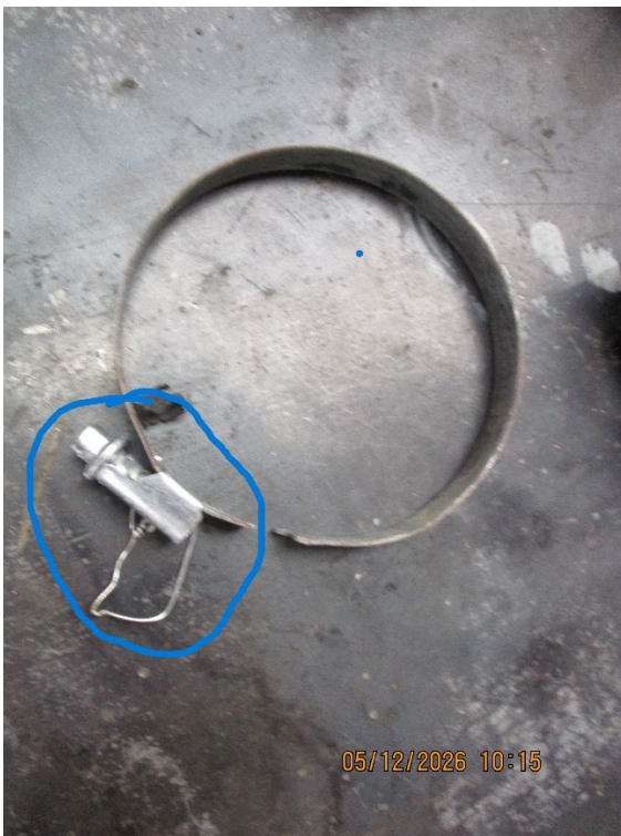
Fig. 8. Disconnected clamp found under intake ductwork. NOTE: screw is worn and loose in clamp housing.
