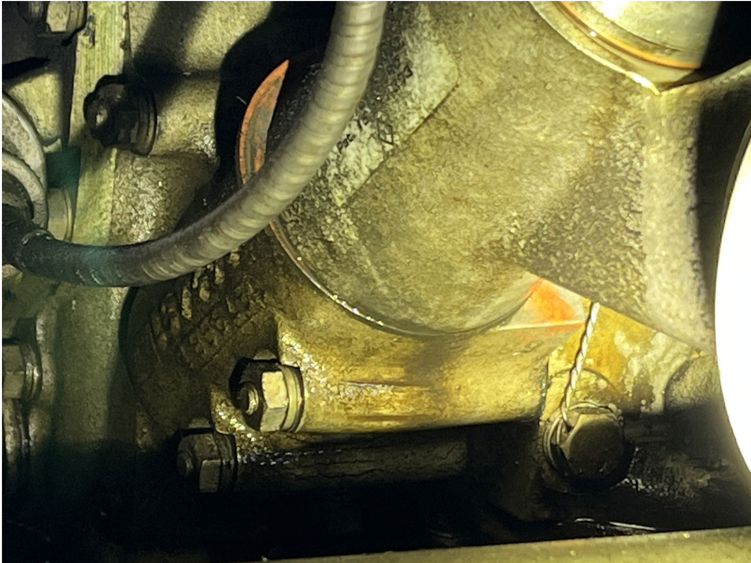
Photograph 3 - Oil filter adapter, Note: gasket protruding and leaking oil (Courtesy of FAA)
