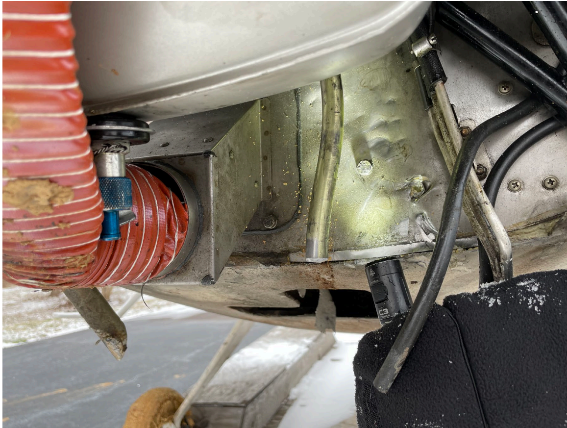
Photograph 4 - Firewall structure accident damage (Courtesy of FAA)
