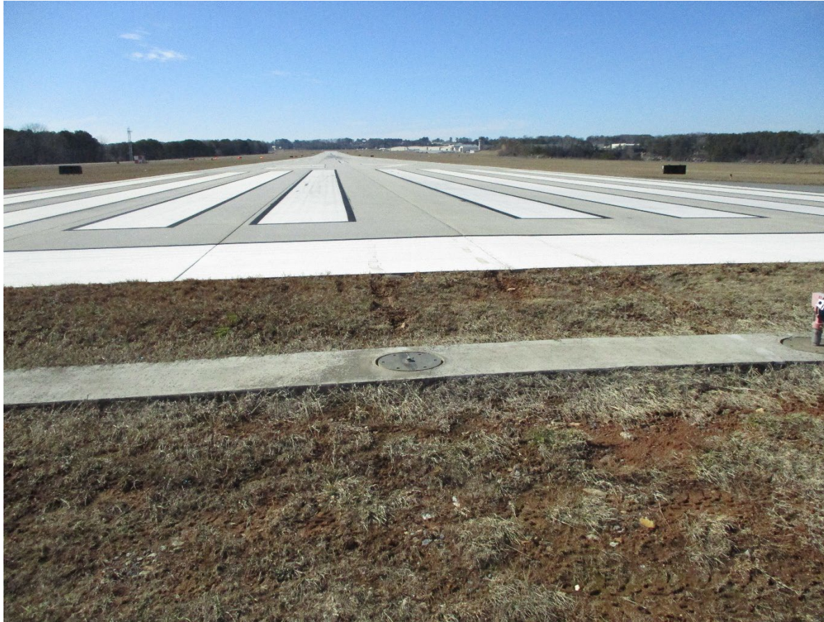
Photograph 2 - Damaged Runway Light (Courtesy of FAA)
