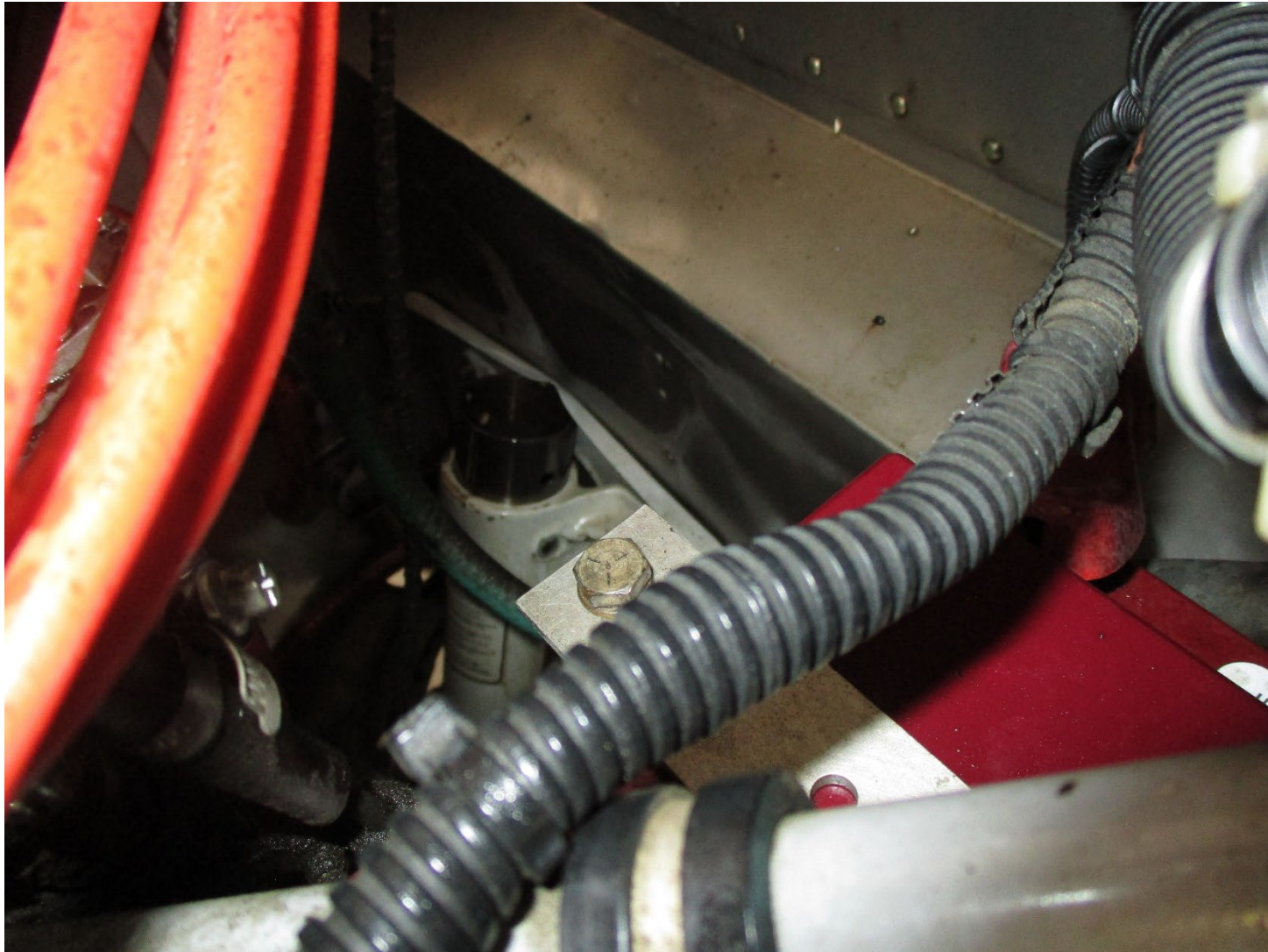
Photograph 3 - Firewall Damage (Courtesy of FAA)
