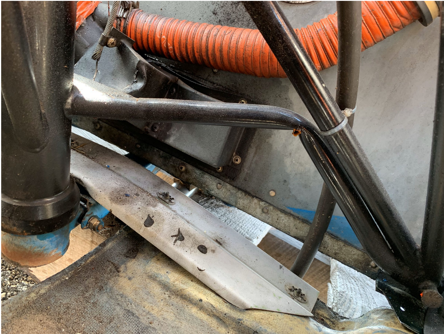
Photograph 4 - Damage to tubular engine mount (Source: SkyBlue Aviation)
