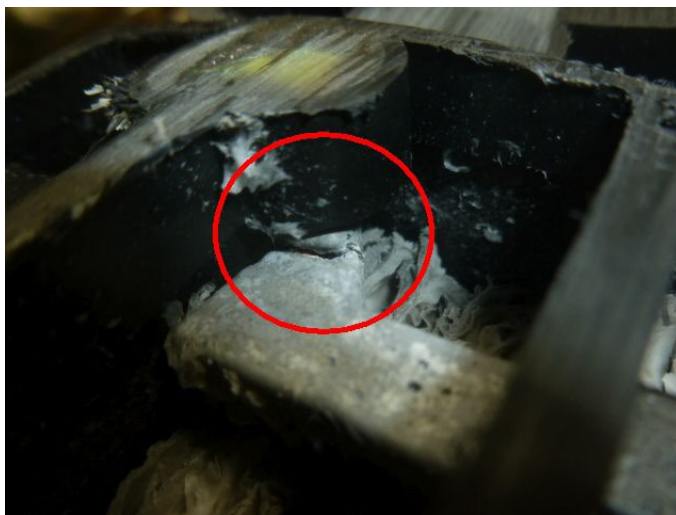
Photograph 4 - Crack in Battery Bridge (Courtesy of Pilot)
