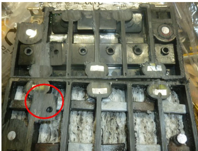
Photograph 3 - Crack in Battery Bridge (Courtesy of Pilot)
