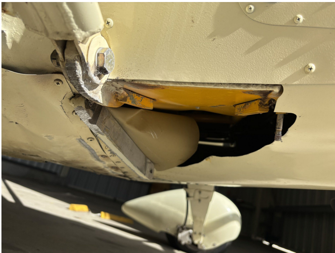
Photograph 6 - Postaccident damaged landing gear attach bracket and lower wing strut attach fitting (Courtesy of Pilot)
