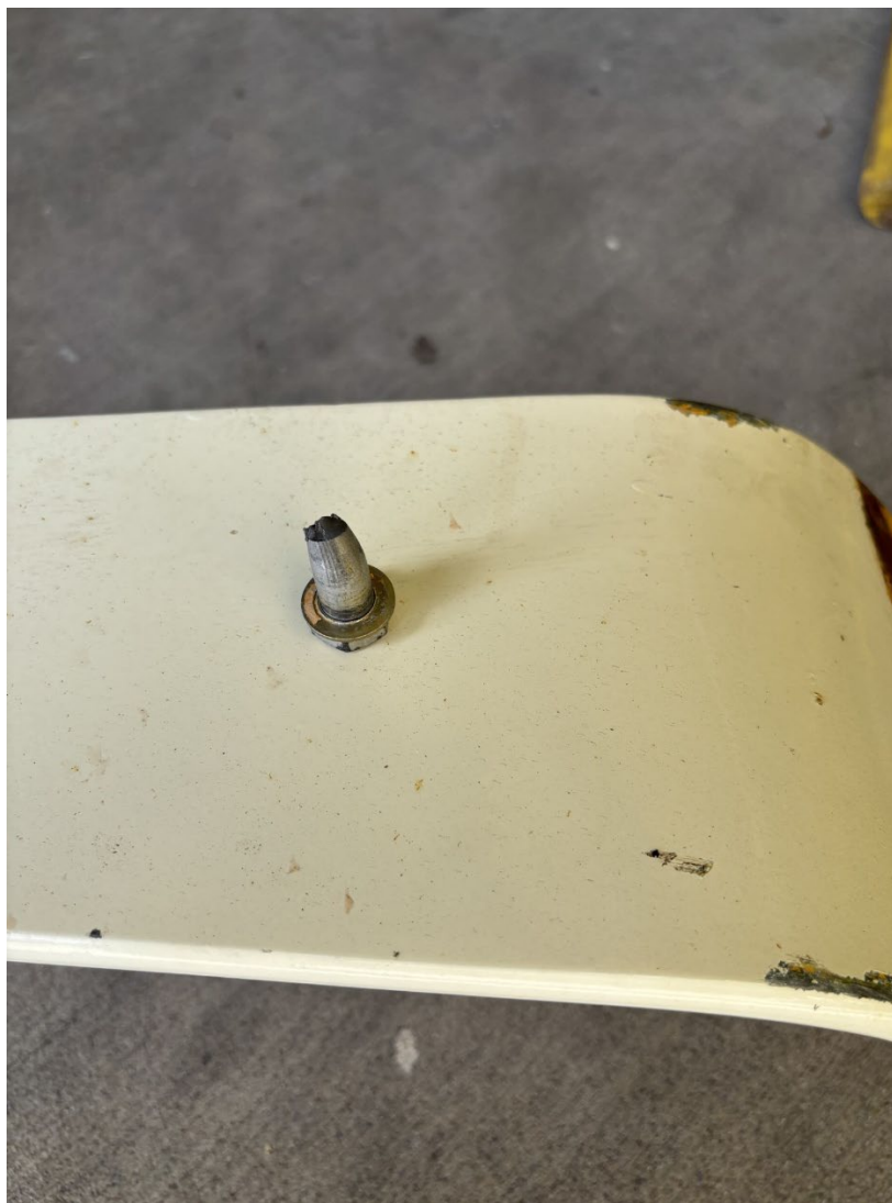
Photograph 5 - Right main landing gear attach bolt half (Courtesy of Pilot)
