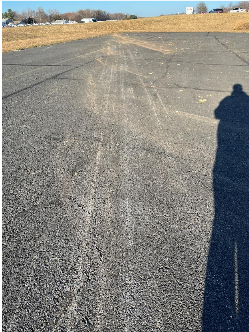
Photograph 5 - Image of ground scars on the tarmac (looking toward runway) (Source: FAA)
