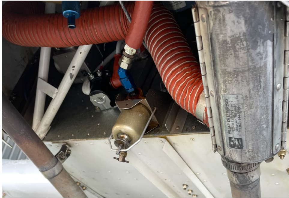
Figure 1 Gascolator/fuel bowl installed as discovered was installed partially outside of the engine compartment.
