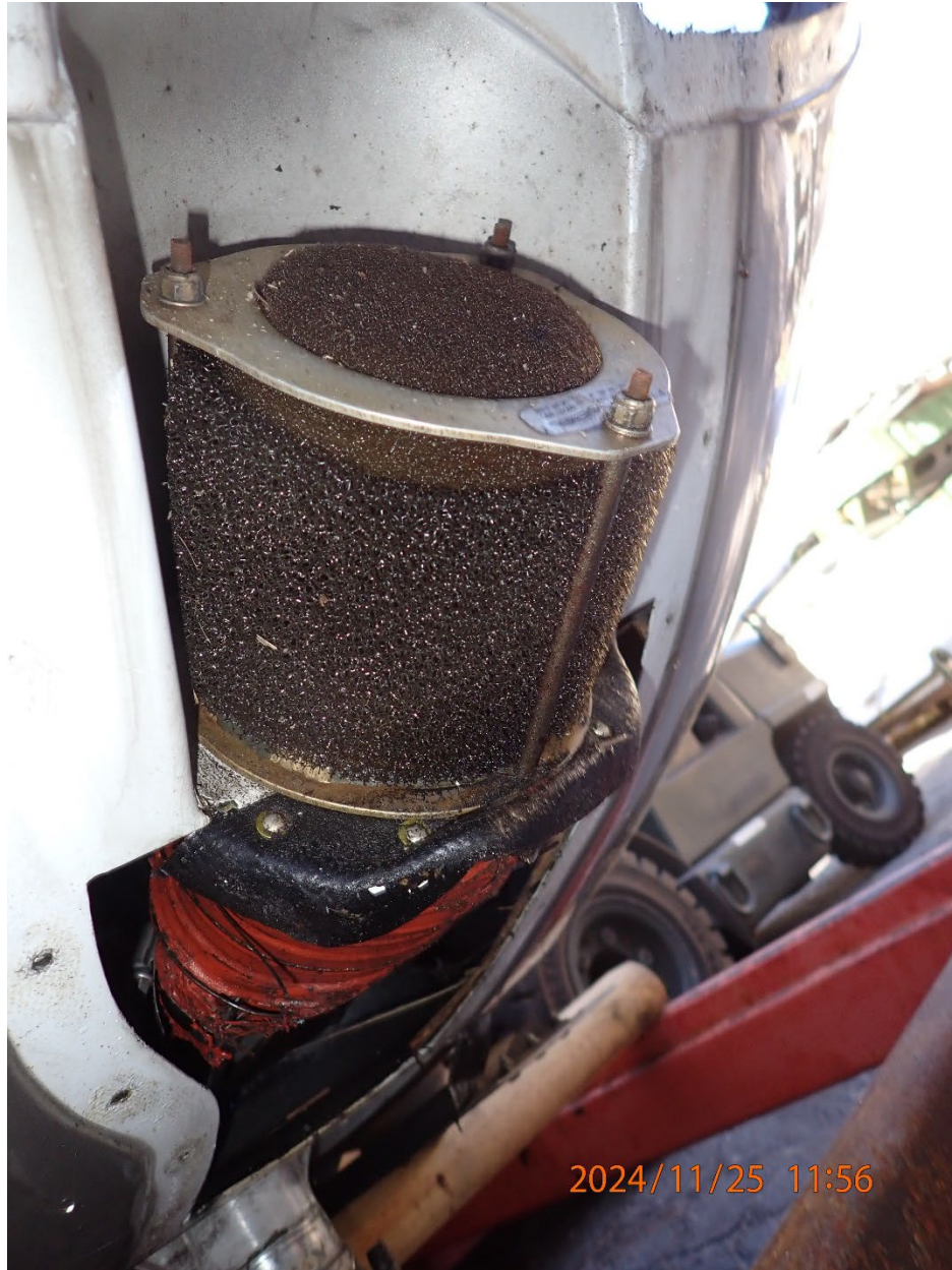
Photo 2: View of the unobstructed engine air intake filter.
