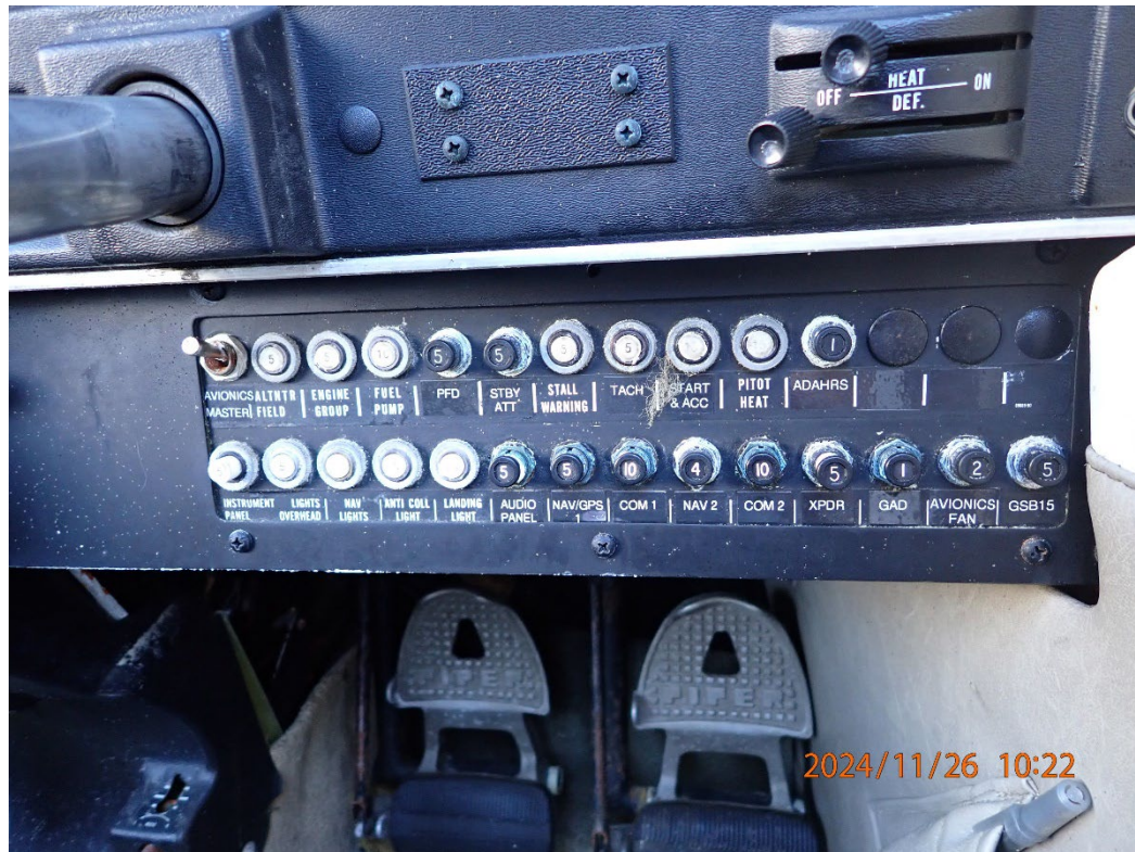
Photo 10: View of the circuit breaker panel.
