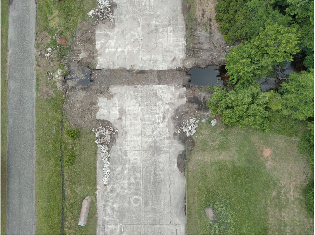
Figure 1: View of the damaged runway. (Courtesy of Nassau County Sheriff's Office)
