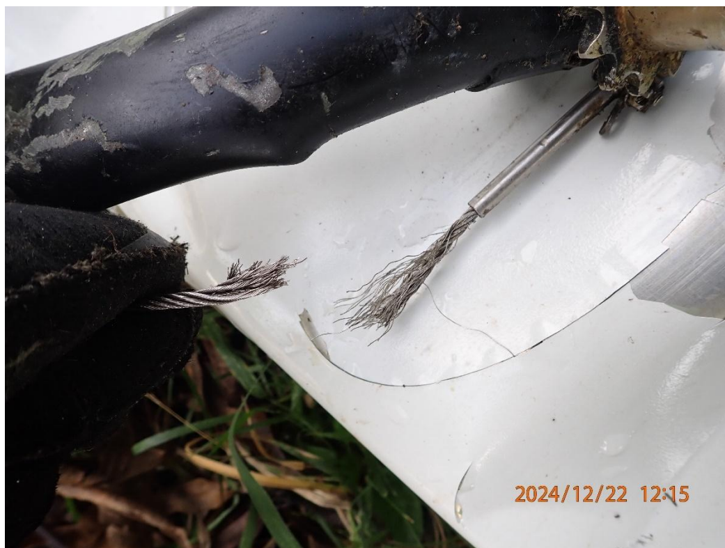
Photo 23: View of the control cable fracture.
