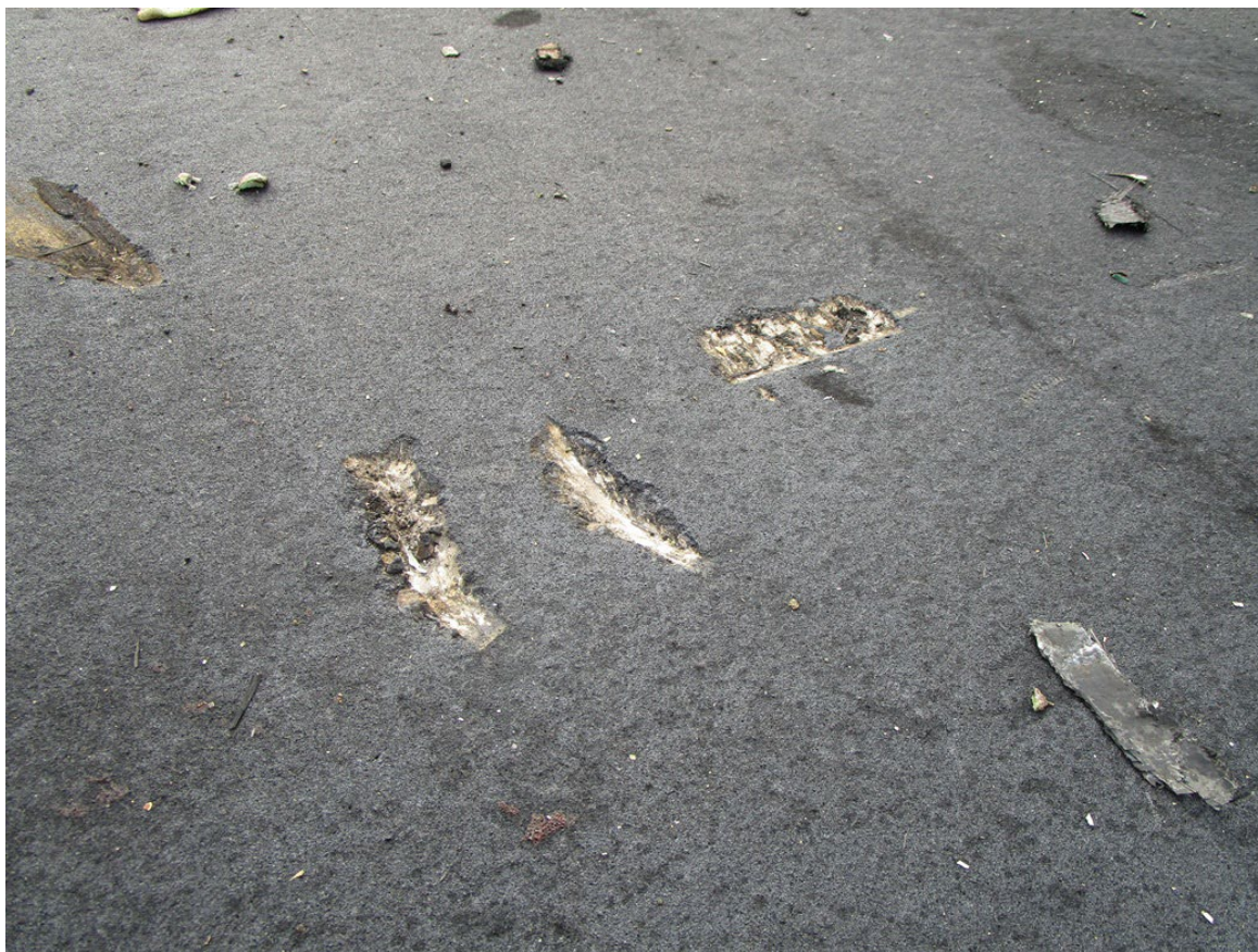
Photograph 4 - Propeller Gouges on Runway (Courtesy of FAA)
