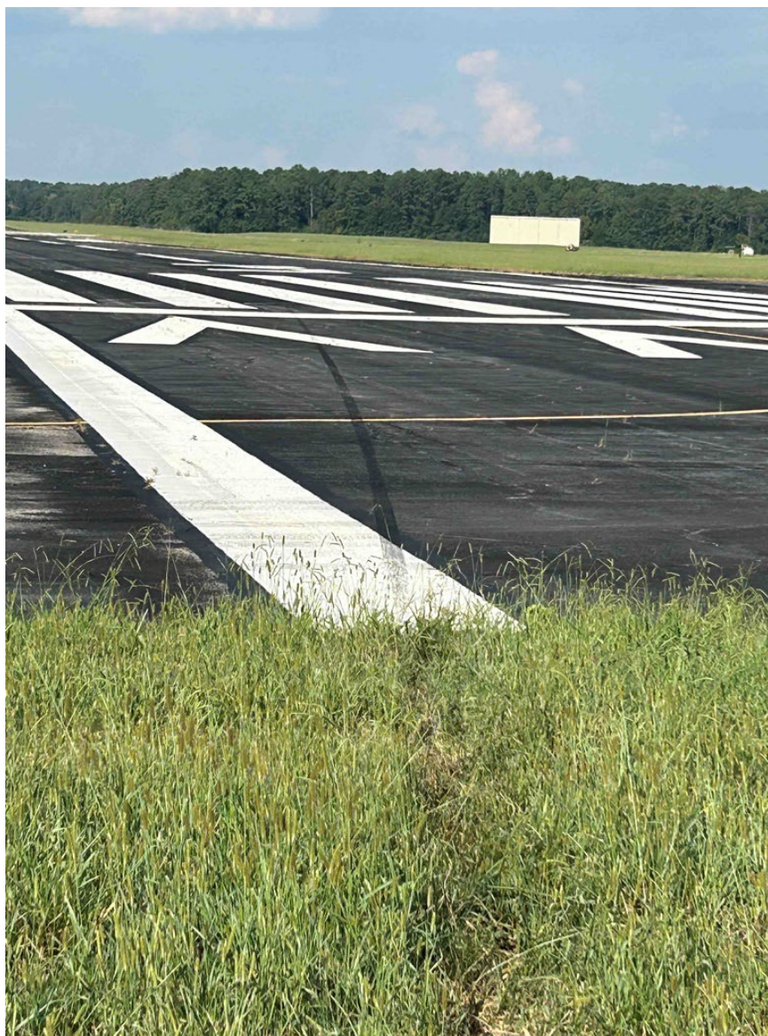
Photograph 4 - Runway Skid Marks (Courtesy of FAA)
