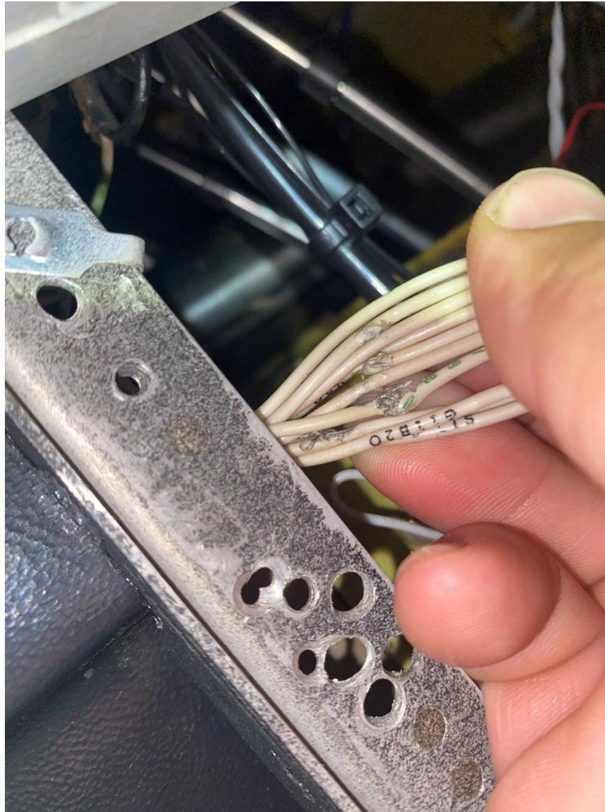
Photograph 2 - Chafed gear switch wires (Courtesy of FAA)
