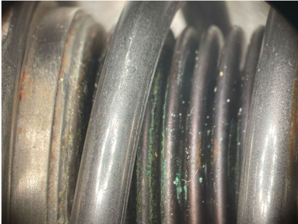
Figure 3: View of corrosion on the bellows assembly. (Courtesy of Woodward)
