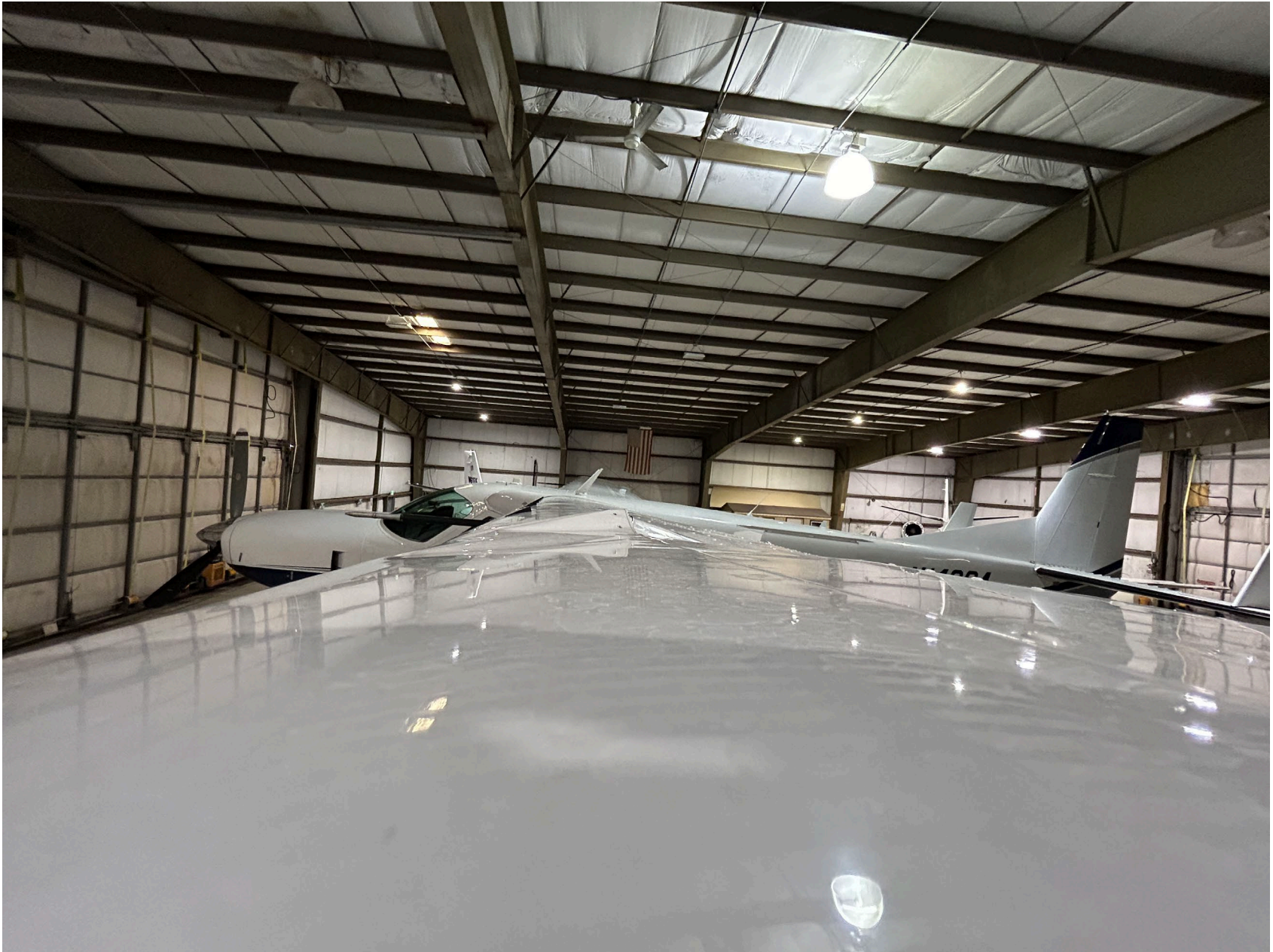
Photo 2 – Top View of Left Wing Facing Inboard (FAA)
