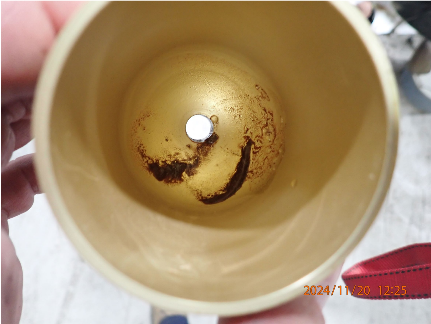
Photograph 4 - Debris is the Bottom of the Fuel Strainer
