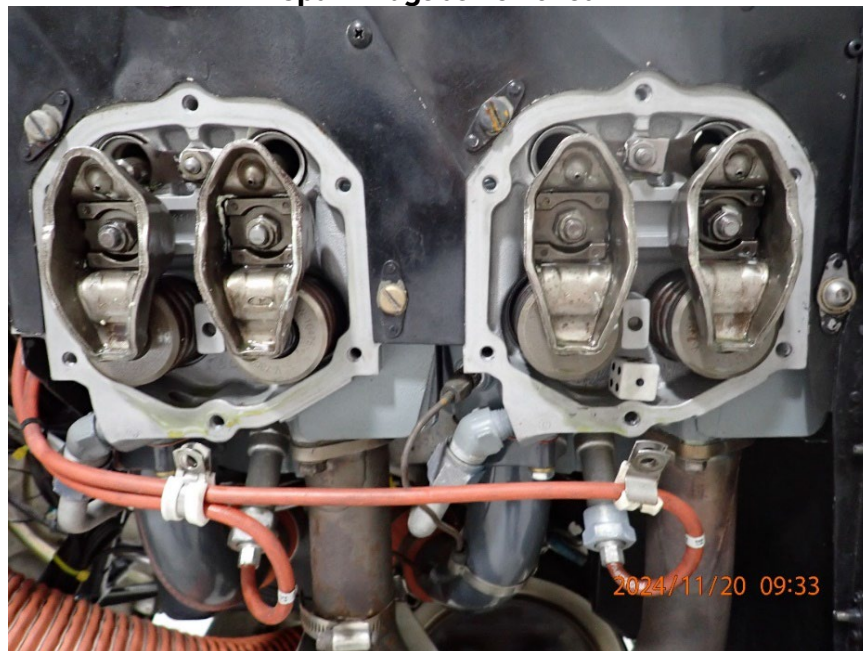
Cylinders 1 (right) and 3 (left) with the Induction Pipes, Exhaust Pipes, and Lower Leads Attached
