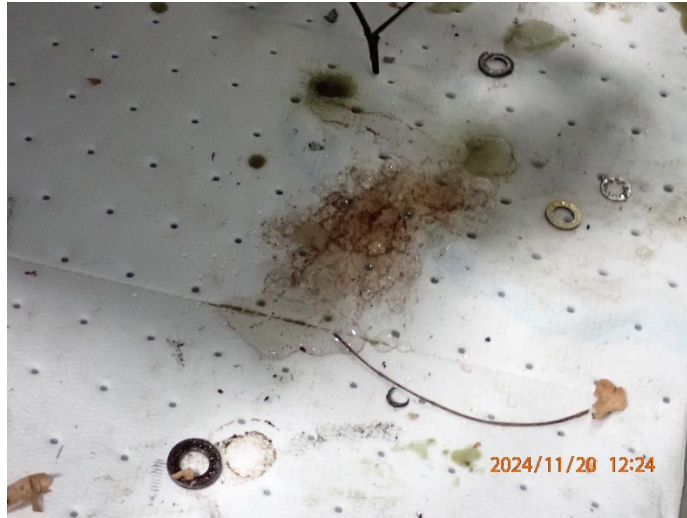
Remaining Liquid and Debris from Fuel Strainer
