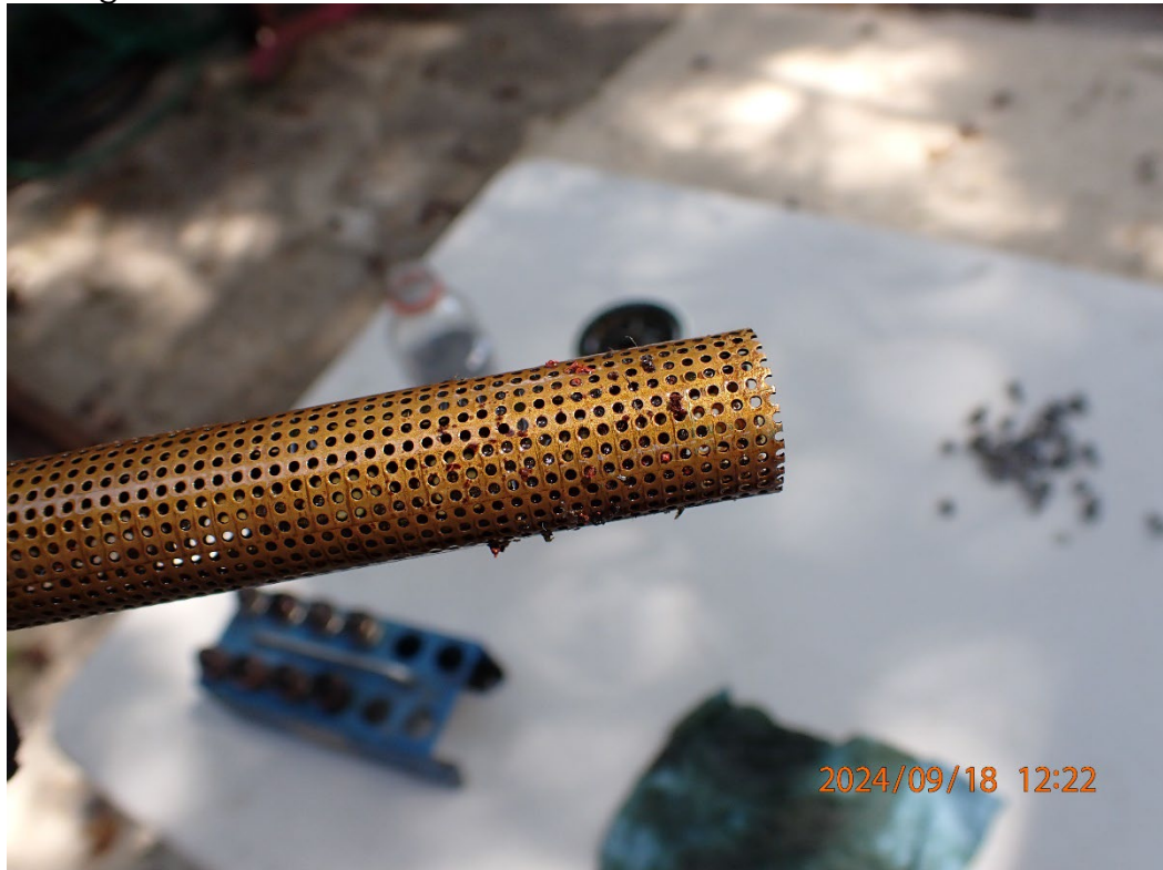
Photo 4: View of the oil suction screen.
