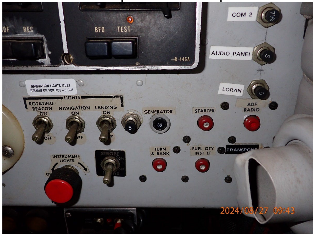
Photo 23: View of circuit breakers and switches.
