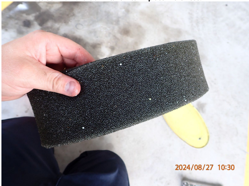
Photo 31: View of the unobstructed air intake filter.
