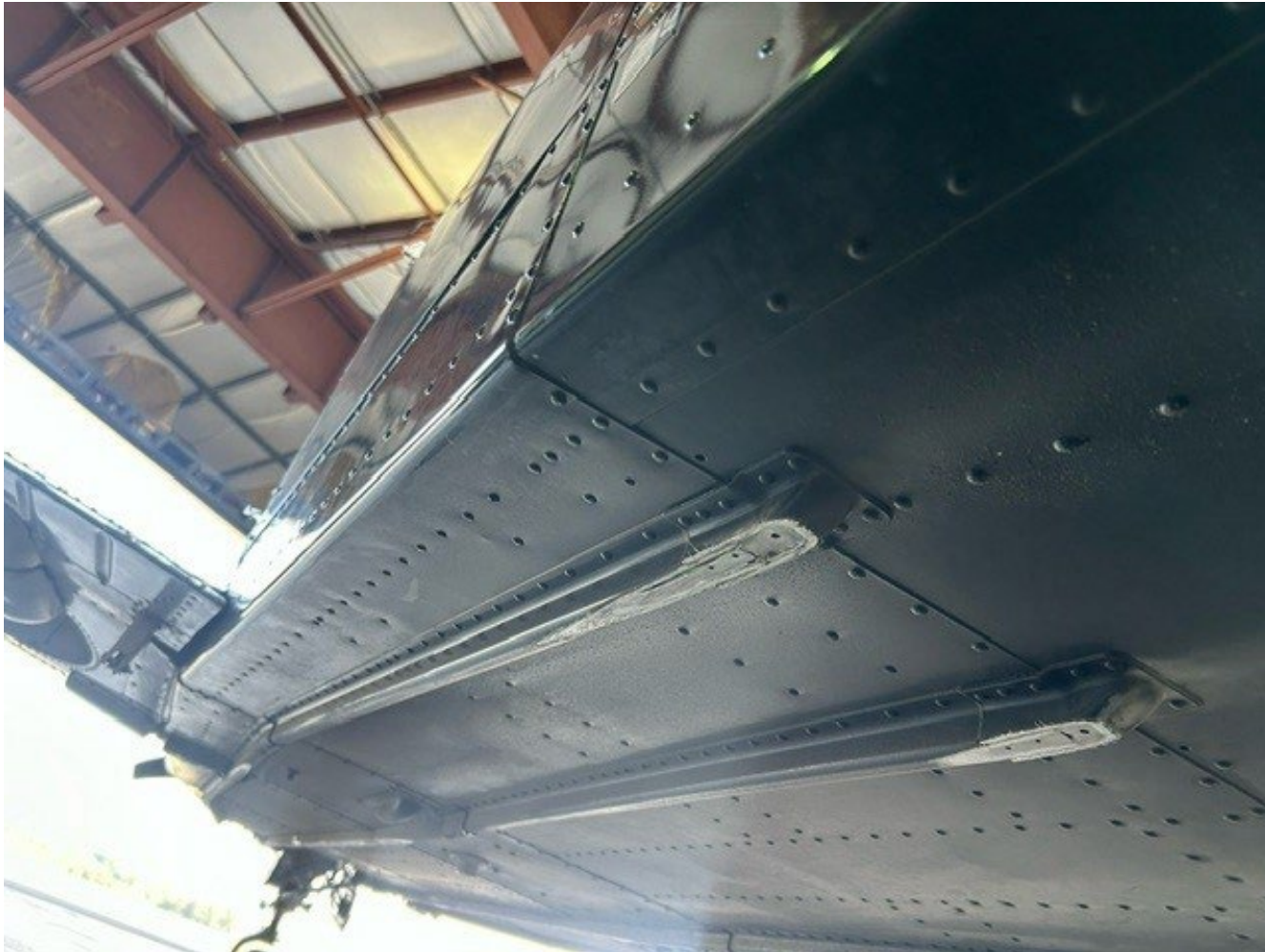
Photograph 3 - Damage to external longerons (Courtesy of FAA)
