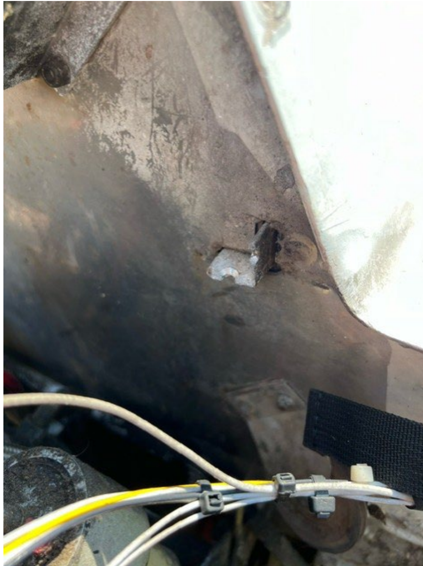
Photograph 3 - Sheared Engine Mount 2 (Courtesy of pilot)
