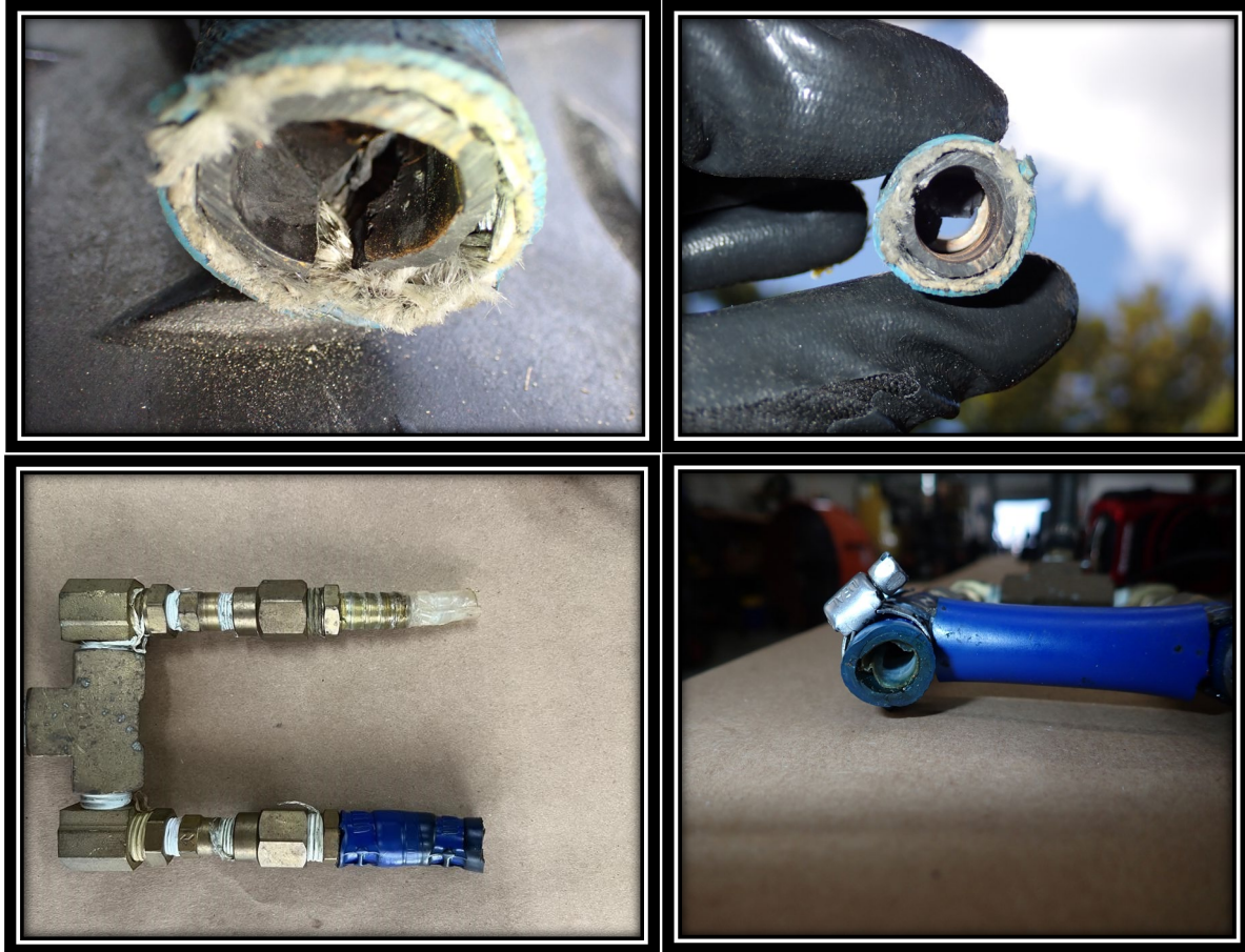
Figures 2 through 5 - Blocked and broken manifold lines for electric-driven fuel pump
