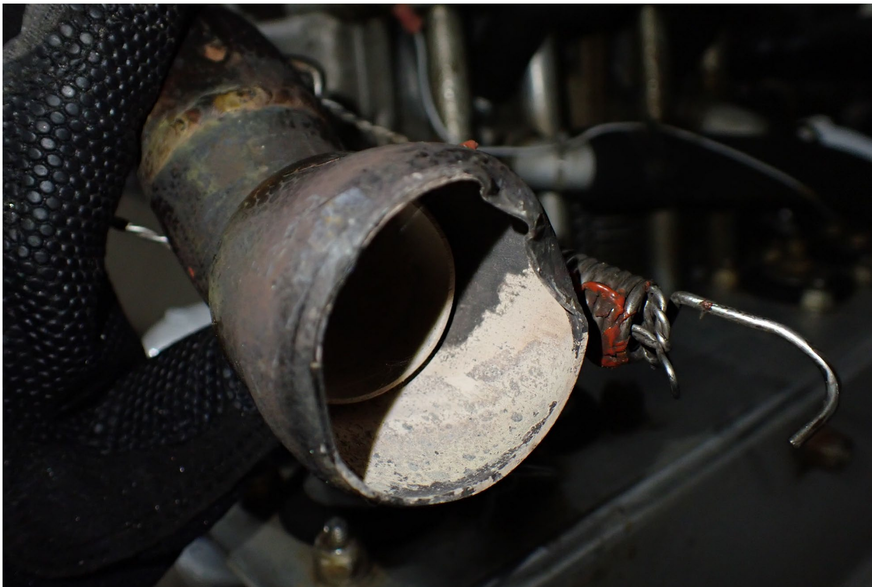
Photograph 12 - No. 2 exhaust riser end
