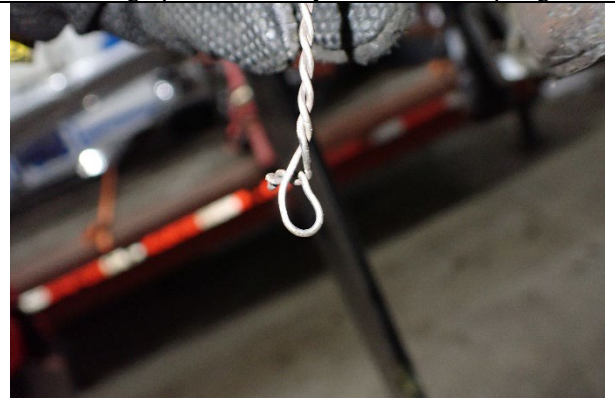
Photograph 29: No. 2 cylinder exhaust riser safety wire
