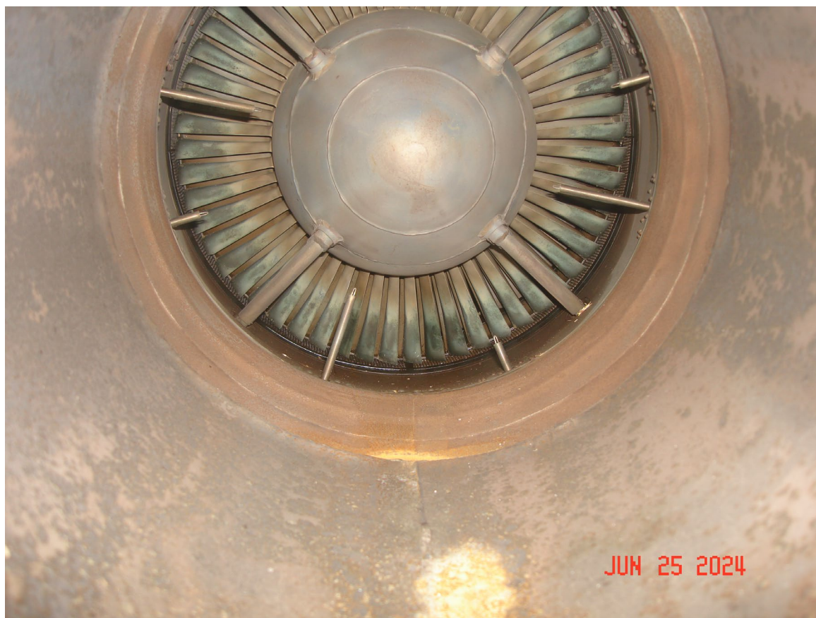
Photograph 6 - Exhaust Area (Courtesy GE)
