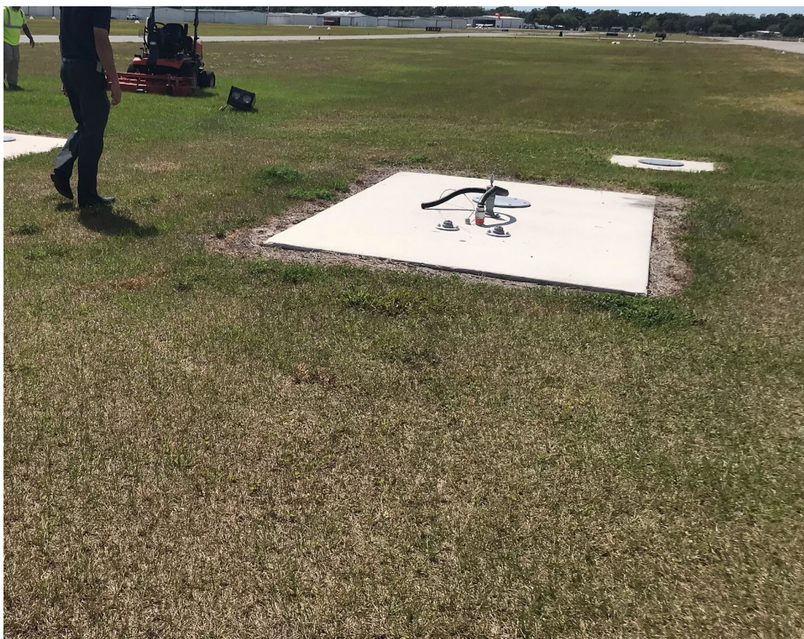
Photograph 1 - Postaccident damage to airport PAPI light (Courtesy of FAA)
