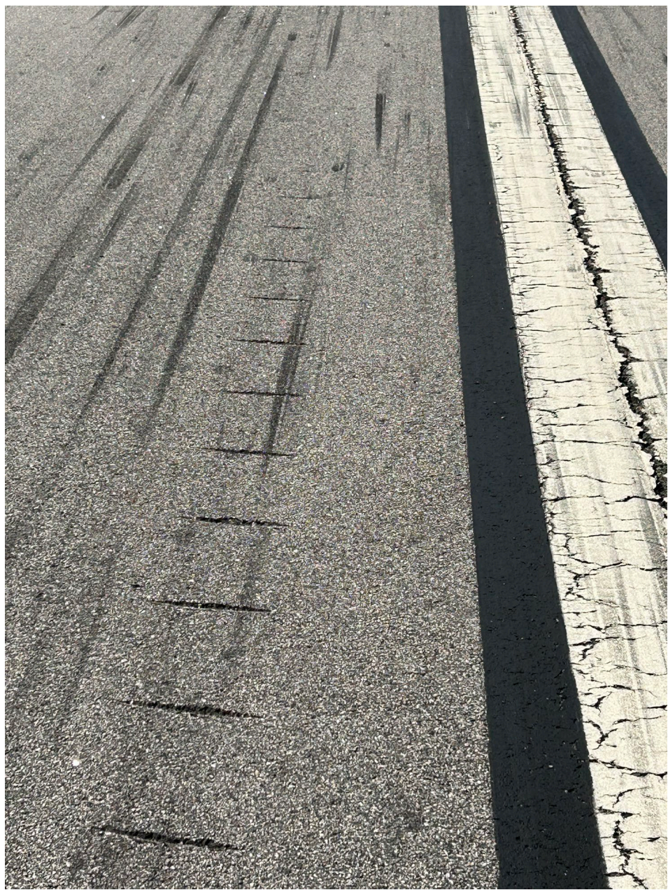
Photo 5 – Close View of Pavement Striations Perpendicular to Runway Centerline (RDU)
