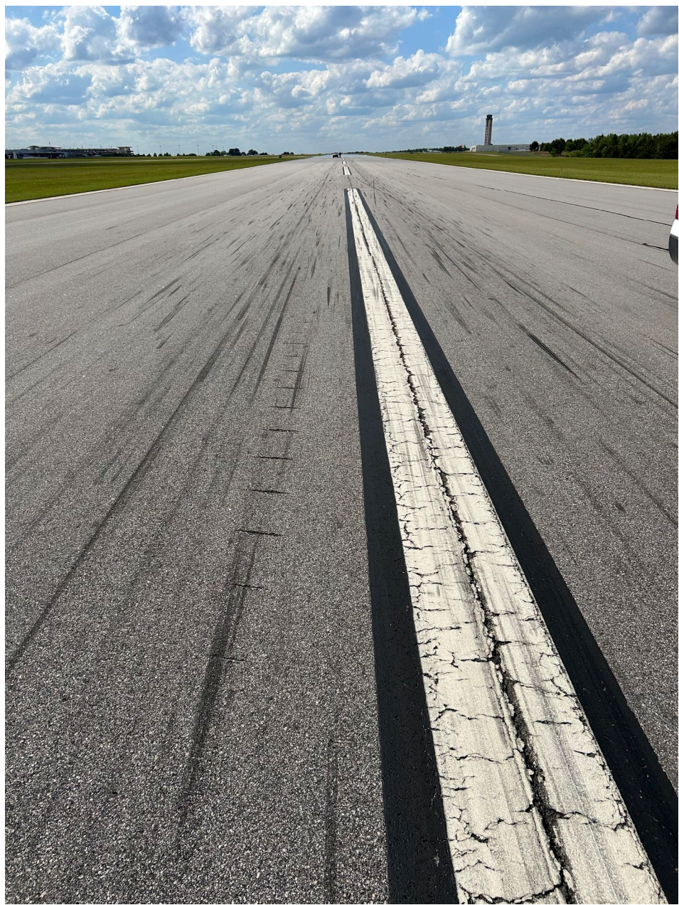
Photo 4 – View of Pavement Striations Perpendicular to Runway Centerline (RDU)
