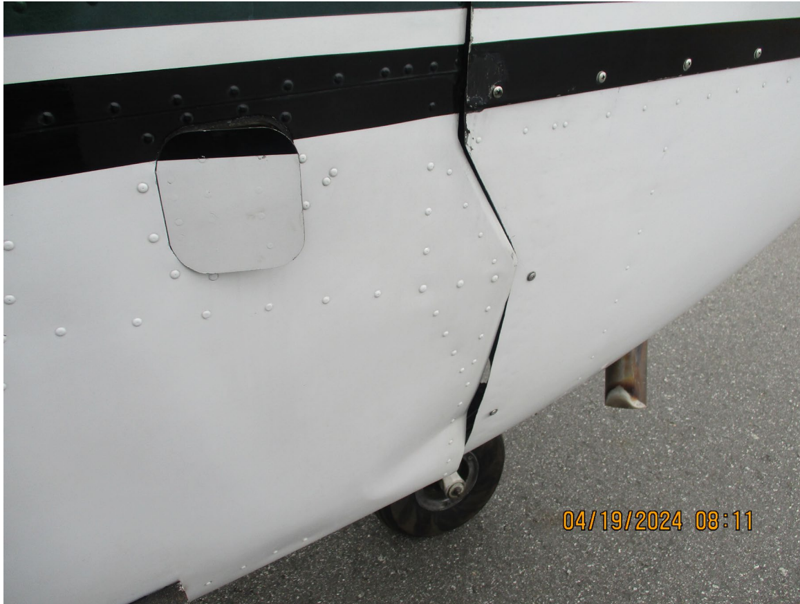
Photograph 4 - Right Angle View of Right Side Firewall / Cowling Juncture (Courtesy of FAA)
