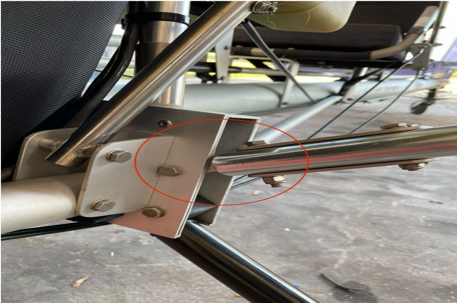
Photograph 8-Wing Connection Point Properly Installed - Non-Accident Aircraft Side 3 (Courtesy of FAA)
