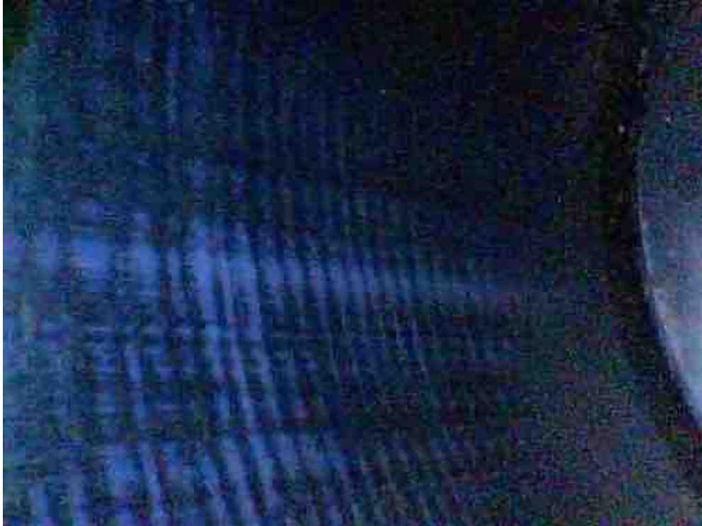
Photo 23 - Borescope photo of No. 3 cylinder wall with circumferential markings.
