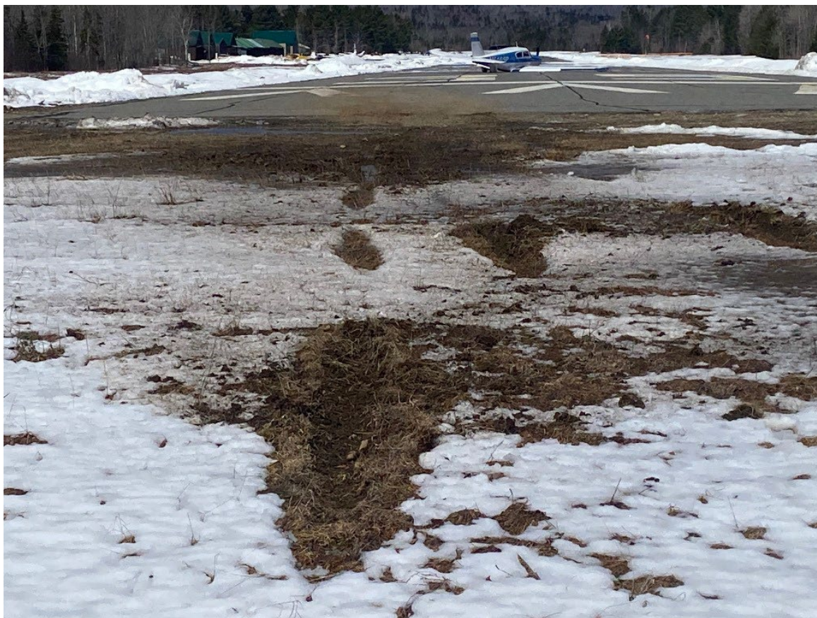
Photograph 1 - Initial Impact Point with Airplane on the Runway (Courtesy of B21 Airport Manager)
