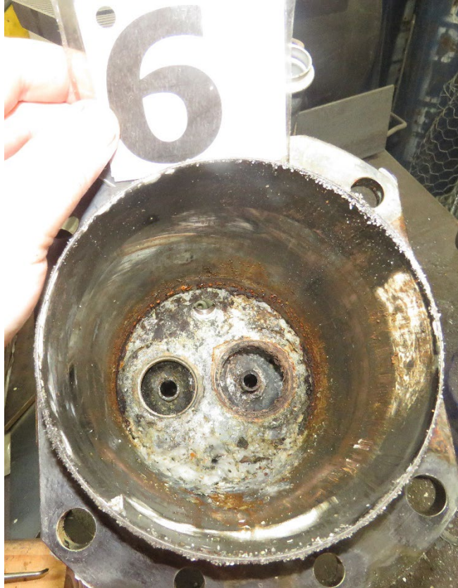
Photo 53 - View of cylinder with valves removed.
