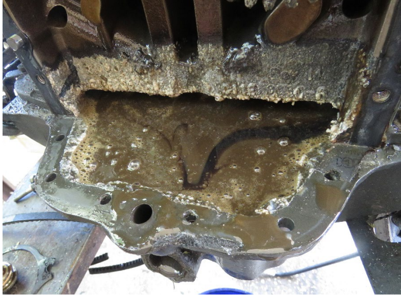
Photo 33 - View of oil sump filled with sludge.
