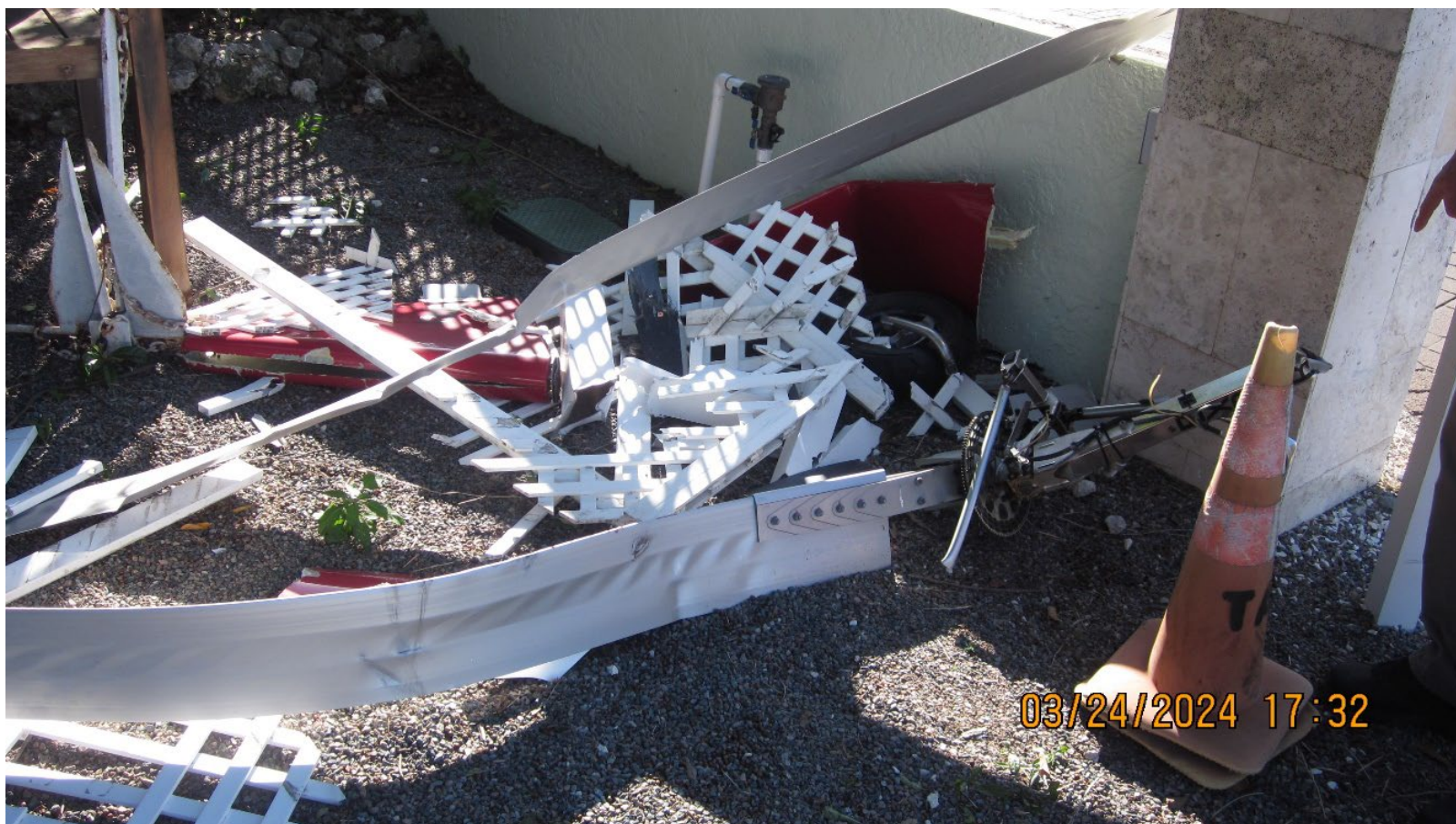
Photograph 5 - View of fence damage and gyroplane debris (Courtesy of FAA)
