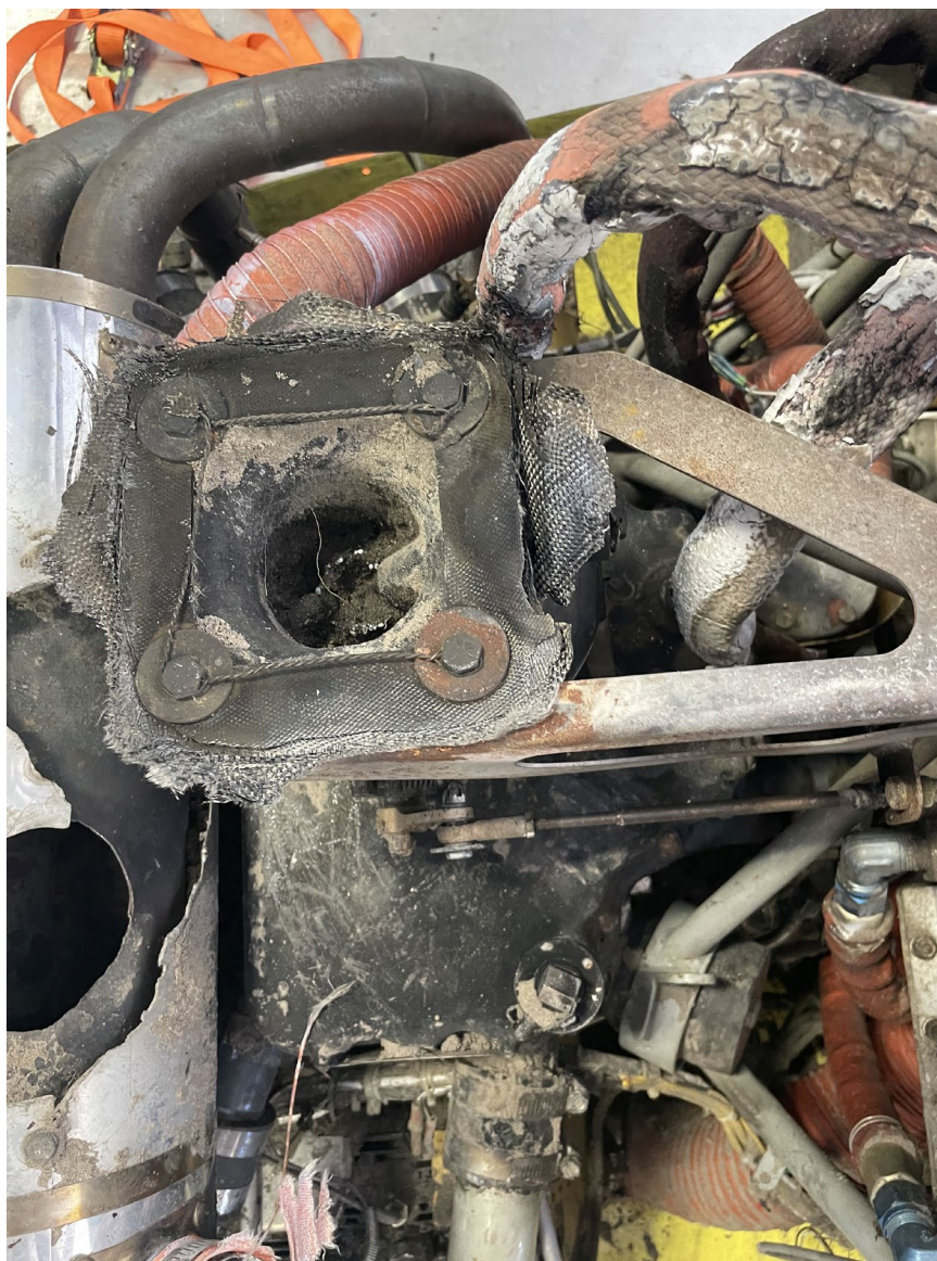
Photograph 4 - Melted carburetor and fuel lines. (Courtesy of FAA)
