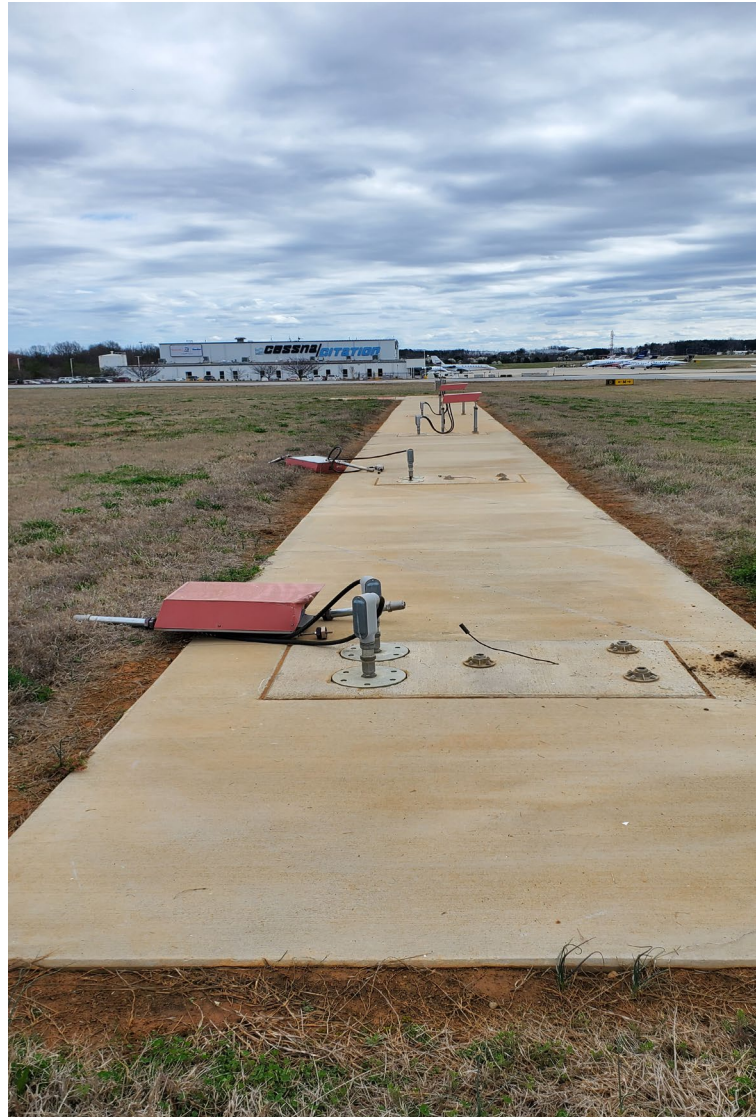
Photograph 3 -Damage to visual glide slope lights. (courtesy of FAA)
